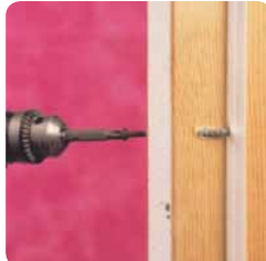
Drywall Screw Piercing Insulation
