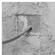
Stucco covering the bracket is chipped away.
