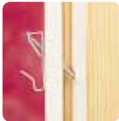
Nails or screws carelessly driven into walls
